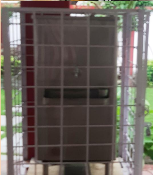
WATER COOLER MACHINE
